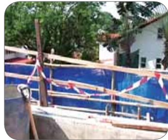
Figure 10: Examples of ineffective barricades.
