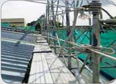
Scaffolds offering roof edge fall protection.
