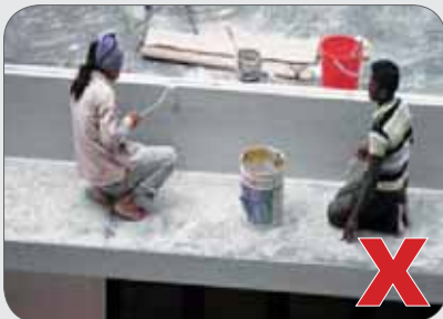
Workers painting near open edge of roof without any fall restraint or arresting systems.
