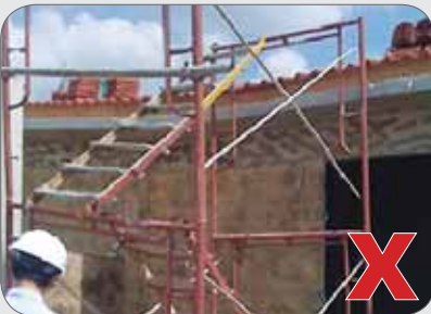
Unsafe scaffold used to access roof.
