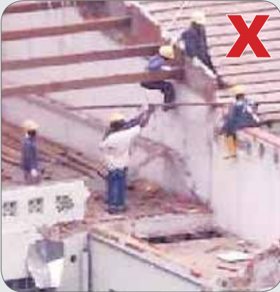
Workers on roof without safety harness with anchorage.
