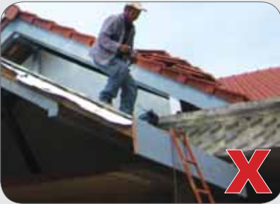
Roof access ladder is not secured to structure at bottom and top rungs.
