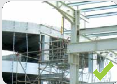
A properly constructed scaffold with hand holds and guardrails for safe access to the roof.
