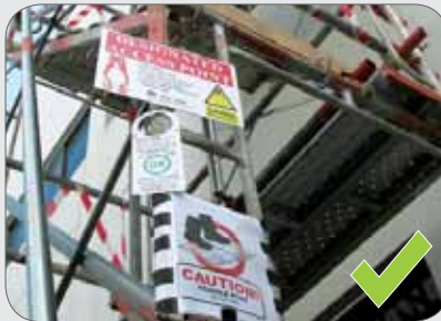
Fragile roof surfaces are identified and warning signage is provided at designated access point(s) onto roof.
