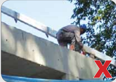
Working on roof without any edge barricade.
