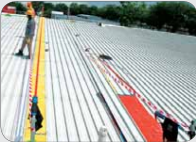
Example of horizontal lifelines on roof.
