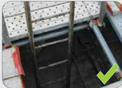
A secured cat ladder with entry opening barricaded.
