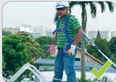
Fall restraint systems used to prevent workers from moving close to edge of roof.
