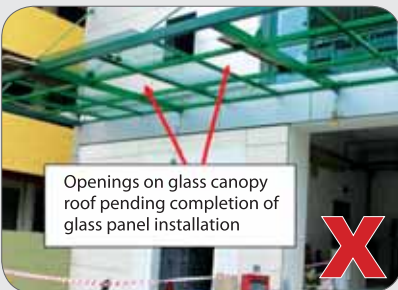
Installation of glass canopy roof without proper access and measures against falling through roof openings.
