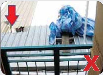
Fragile roof surface is not identified before work and no safety signage is used to warn workers of hazard.
